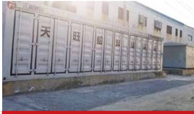
Jiangu Shuyang Energy Storage Project 0.6MW/4MWh
