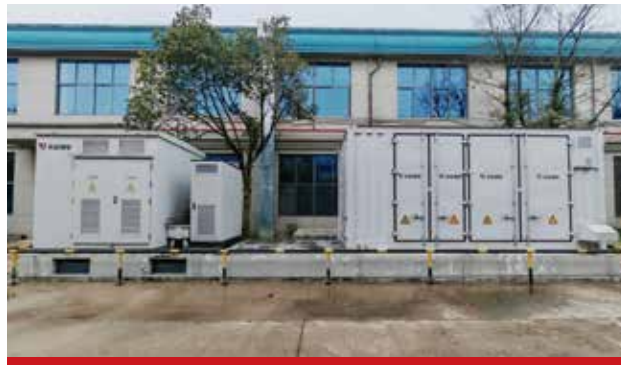
Tianneng Battery Group Headquarters Energy Storage Project 5MW/10MWh
