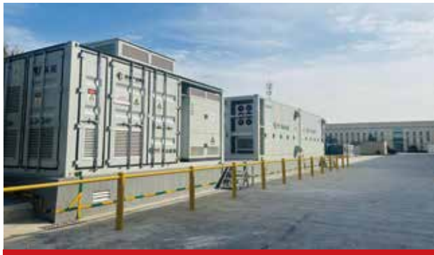
Huzhou Production and Investment Energy Storage Project 10MW/20MWh
