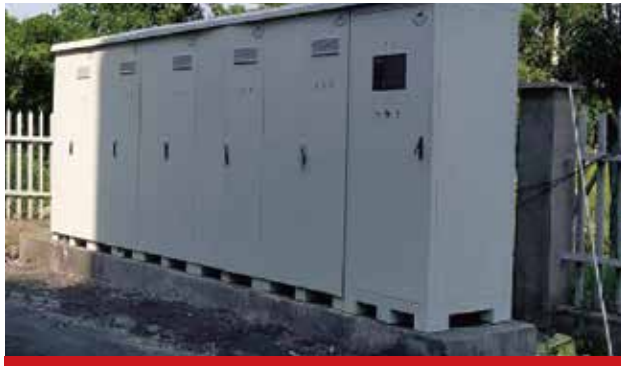
MIZUDA Group Energy Storage Project 1MW/2MWh
